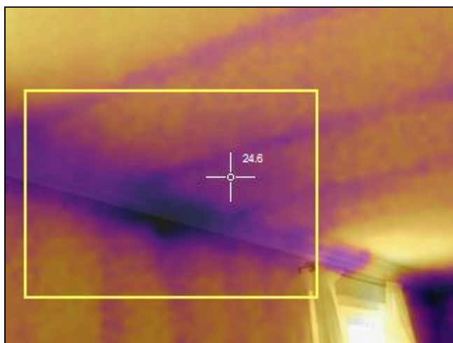
3.1 Item 1(Picture) Master Bedroom Ceiling above bed
