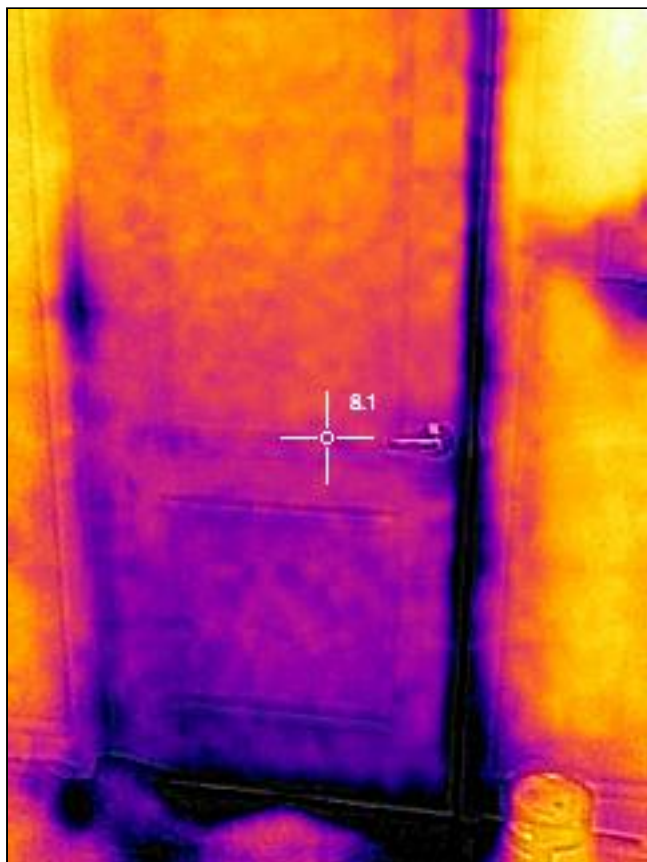
2.3 Item 2(Picture) Cold Room Door - Basement - Heat Loss
