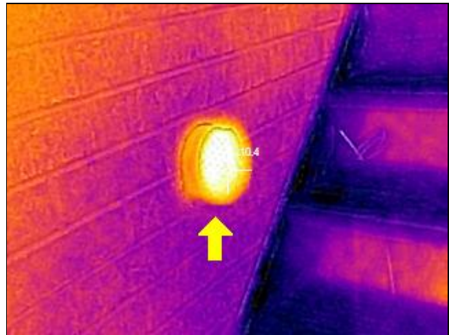
2.1 Item 2(Picture) Missing Vent Cover - Stove Vent
