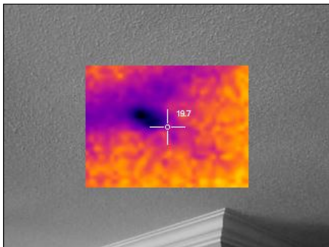
4.1 Item 1(Picture) Thermal Anomaly - Front Bedroom Ceiling
