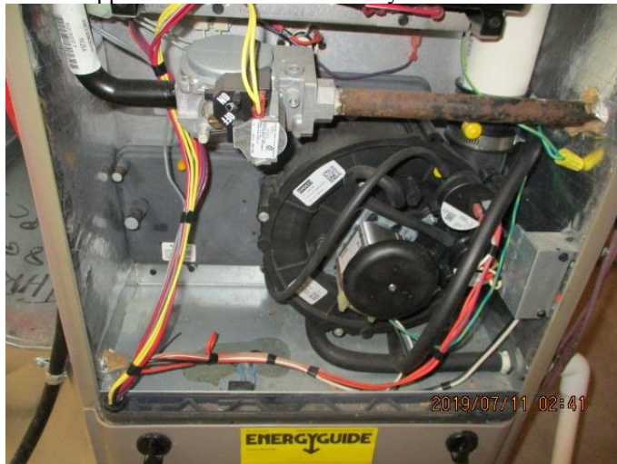
Gas shut off and electrical disconnects provided.
